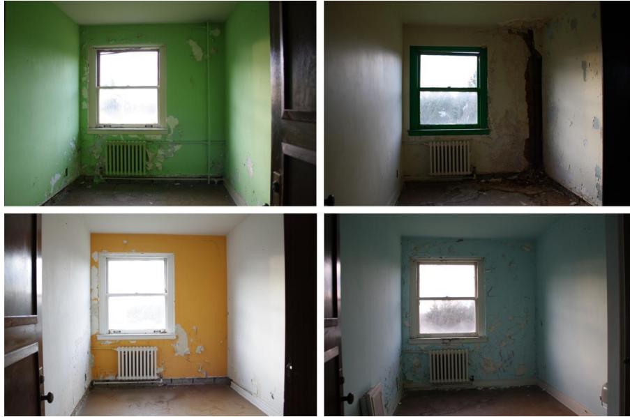
Seminarians occupied tiny rooms. These rooms received their colorful paint when a youth conservation group occupied them in the late 70s. Several small rooms will combine to make a modern hotel room, but door spacing in the hallways will not change.
