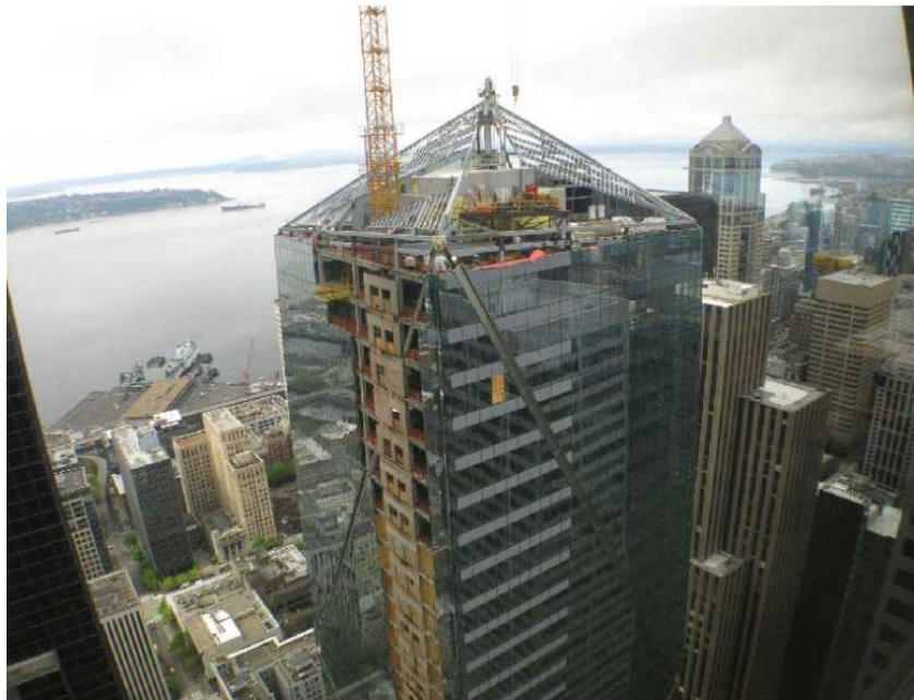
The Mark tower, now F5 Tower, is under construction now. (The Mark Photo)
